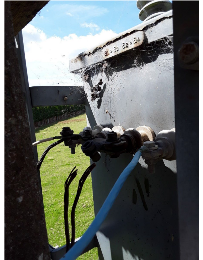
Two earth wires disconnected from central neutral terminals
