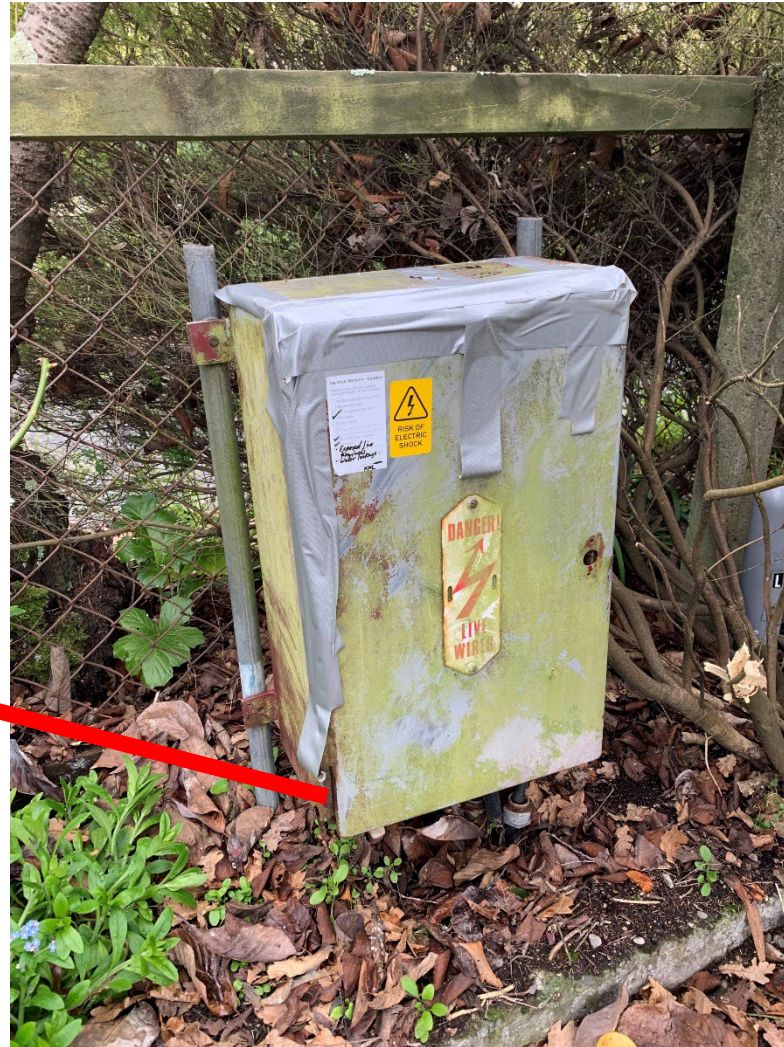
External distribution board
