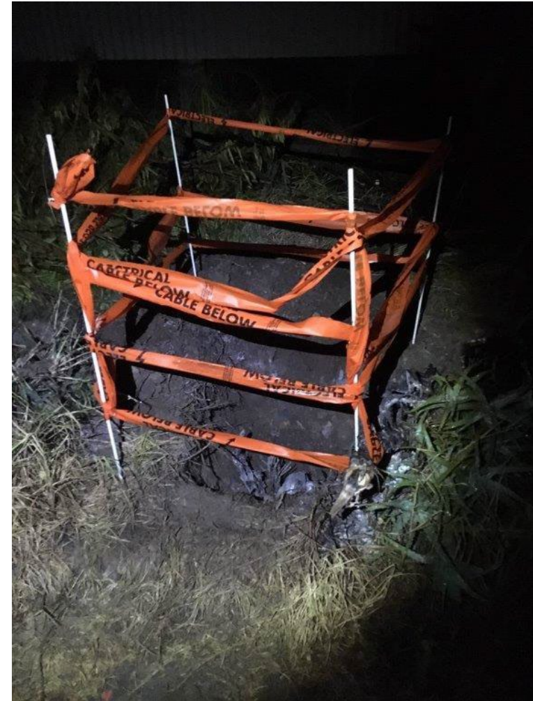
Distribution Pillar fire
