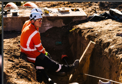
Anchor Block for Ducting at Portobello
