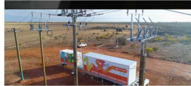
Battery Energy Storage Solutions
