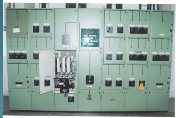
400V circuit breakers (1988)
