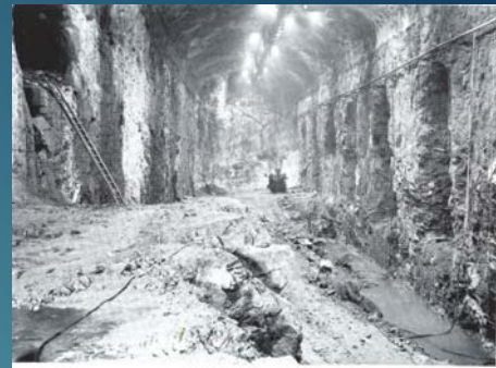
Madapouli Power Project West Arm Powerhouse Contract Excavation in progress in machine hall. View looking West towards emergency exit, with transformer vault excavations on right and ramp from access tunnel to Elev. 5.0 in left background. July 1967
