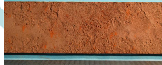
Figure 3 - Bar E Metal loss 1.19mm
